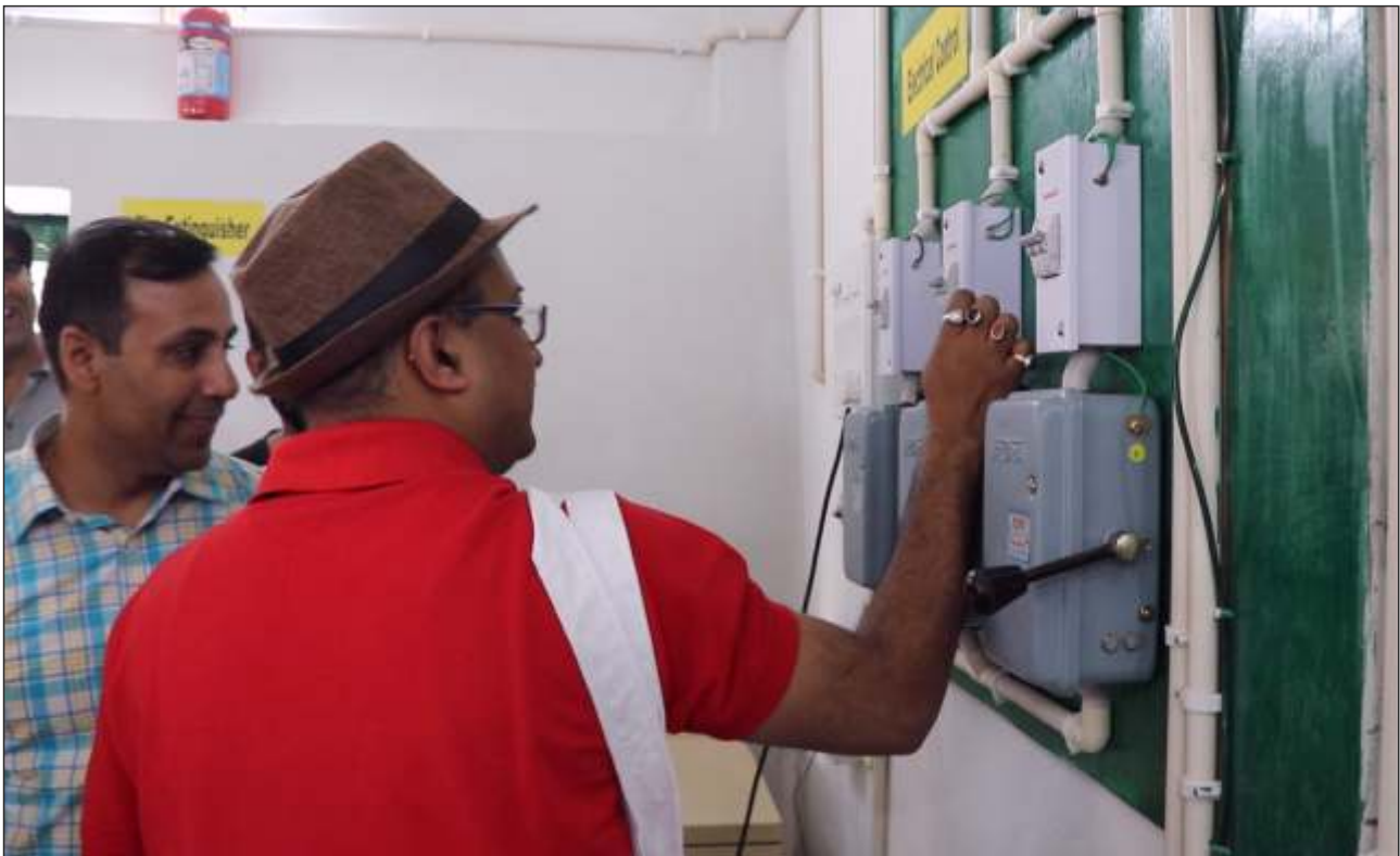
Project LCC member from HSBC switches on the solar panel of the water treatment plant.
